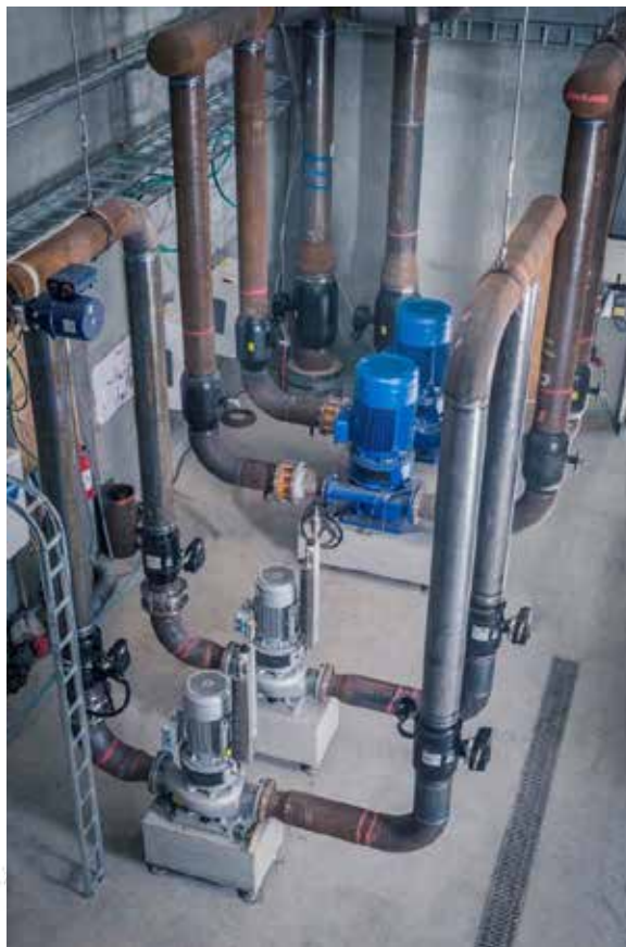
Hobro District Heating Station: Booster station with BROEN Ballomax® valves
